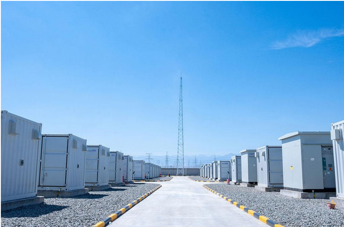
Industrial energy storage illustration | Sunergy
